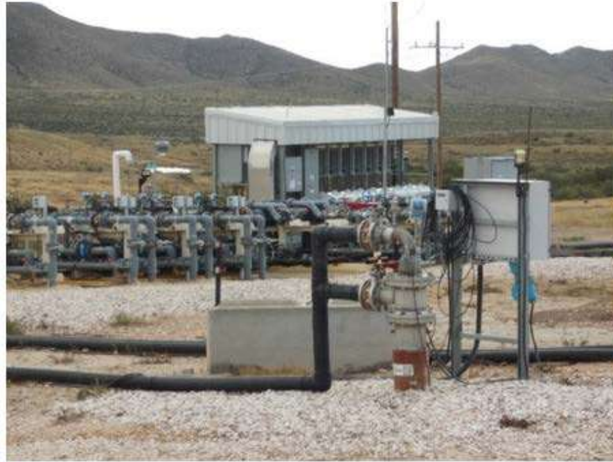
Gunnison wellfield: Wellhead (foreground), valve skid (middle ground), and VFD skid (background)
