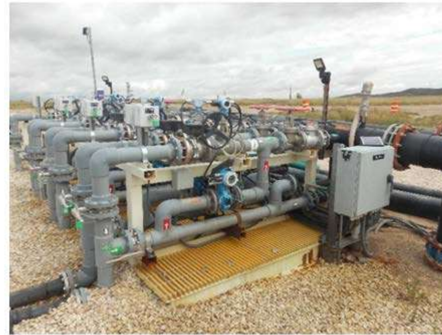
Valve skid detail showing piping manifold and connection to main PLS and raffinate pipelines.
