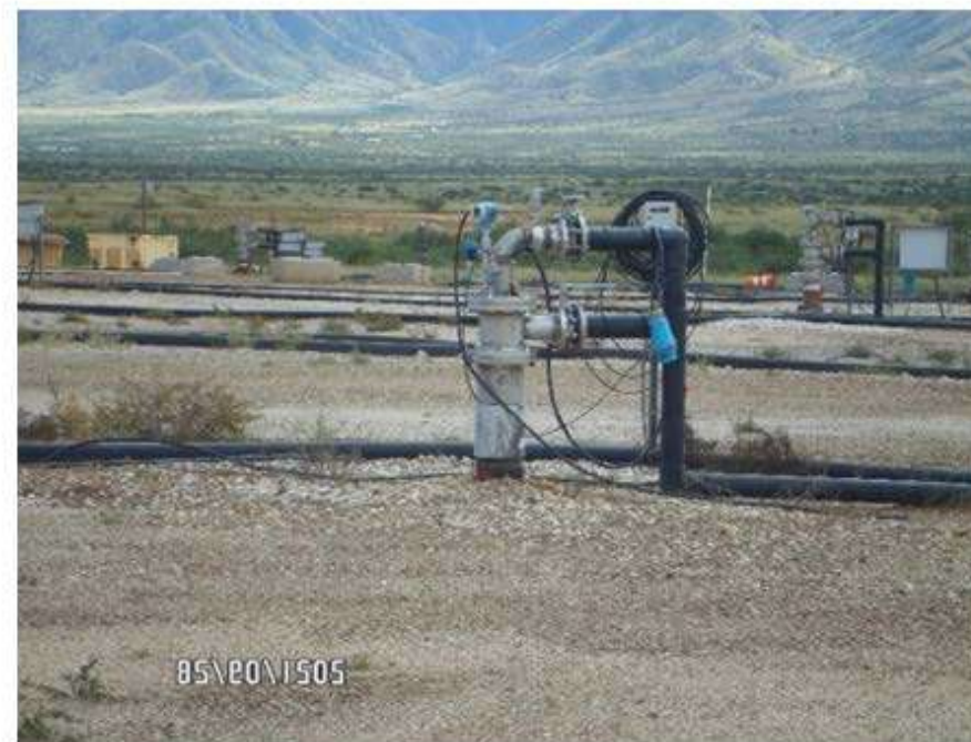
Reversible wellhead showing raffinate and PLS pipeline connections instrumentation, and valving
