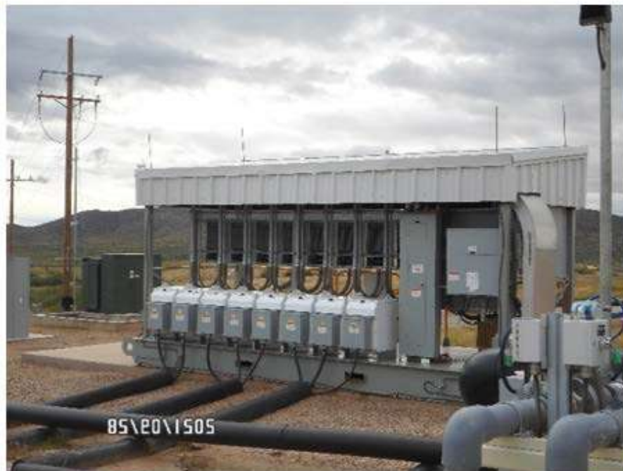
VFD skid detail showing switchboard, distribution panel, VFDs, and exit cabling to wells
